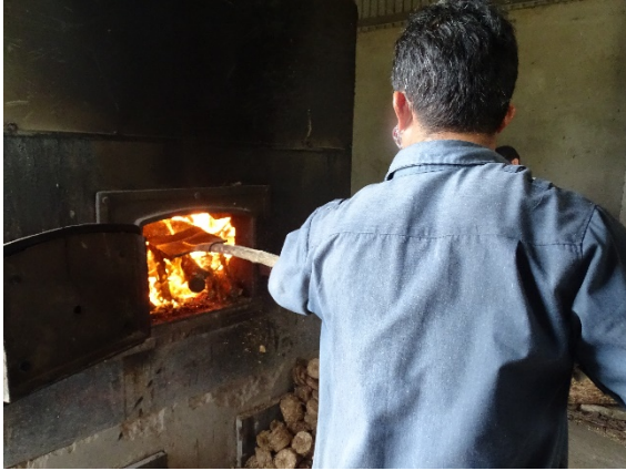
Photo 11. Industrial scale cook incinerator at rubber factory
