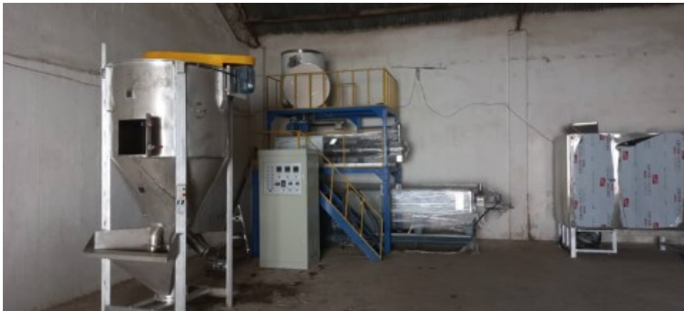
The equipment that was purchased during the project and used to make floating fish feed. Photos taken by Kigen Compton during installation
