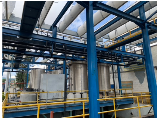
Logstor Industry pipe run 6 meters up underneath the CSP throughs. Installed 50% faster than expected. Picture by Eg Andersen
