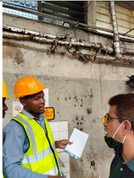
Inspection at Spin Knit factory in Nakuru with SN Technical Director and QUAD management. Picture by Leonard Akohi
