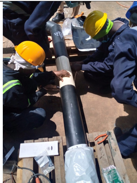
Eight installers from three different companies being trained in installation of fittings, pipes and joints at the training facility. Picture by Eg Andersen
