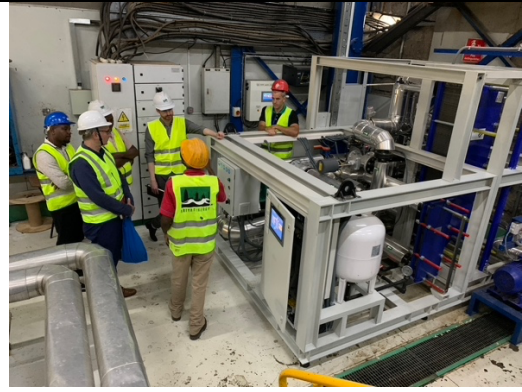
Inspection of heat collector at Iber Africa with NCF, Ariya, IA management and EA Energy. Picture by Eg Andersen
