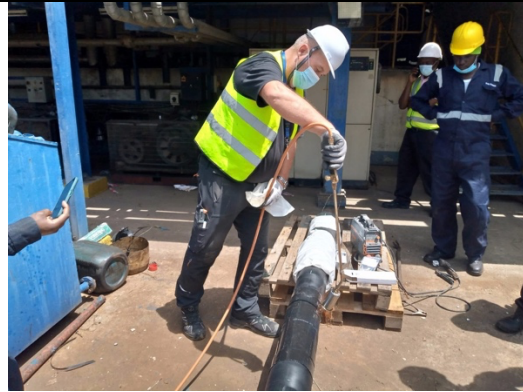
Logstor Academy Instructor Mr. Morten Chemnitz showing how to prepare the installation of a Logstor shrink joint at Iber Africa. Picture by Eg Andersen
